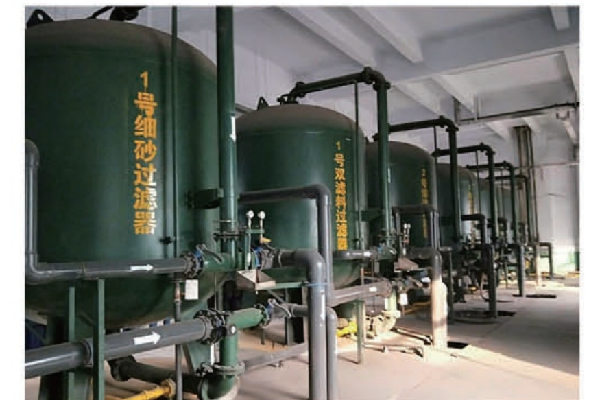
Oxygen plant water treatment workshop
