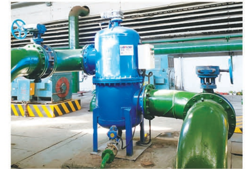
Paper Mill Circulating Water Filtration System
