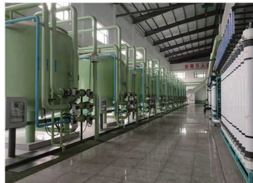
Reverse osmosis pre-sand filter in a chemical plant
