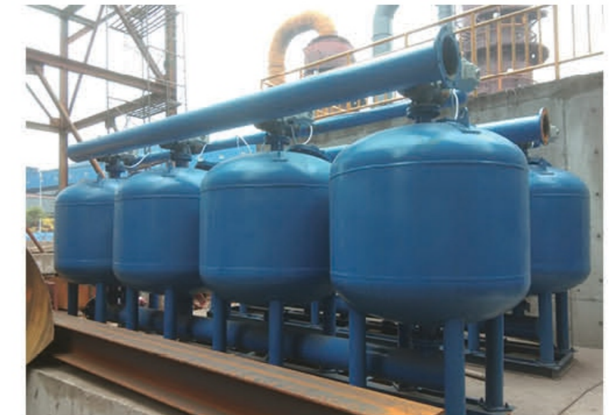
Installation site of a power plant circulating water system
