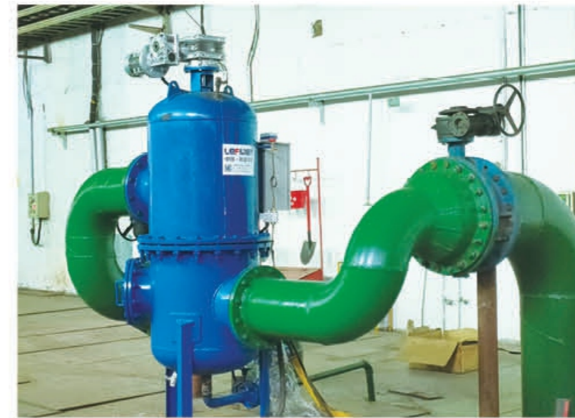
Clean ring water system for steel mills
