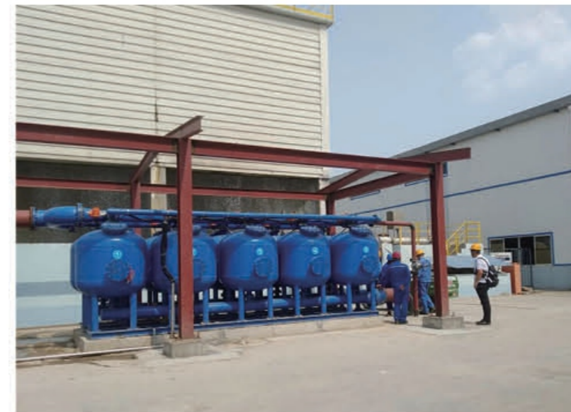
Cooling circulating water system in petrochemical plant
